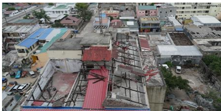
Figure 1: Destruction by TC Idai in Sofala province capital, Beira
